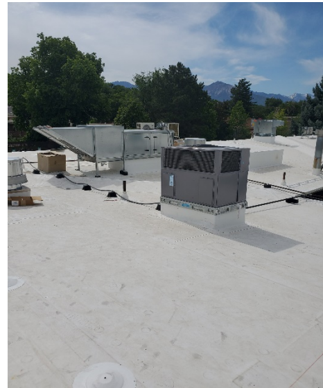
The new roof with cooling/ heating units installed
